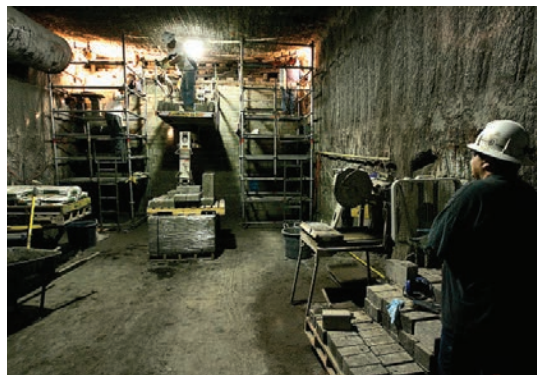
Salt of the earth: Men work to seal a salt tunnel in the Carlsbad Waste Isolation Pilot Plant.
